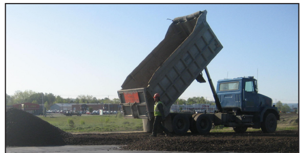
Figure 8. CMV and MDP 40 spatial maps after final pass – TB9b gravel subbase material production compaction (highlighted area subjected to truck traffic carrying/dumping the base material)
