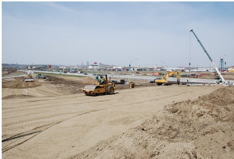
Figure 1. The location of the new bridge during stage 1 (looking west from the existing bridge)
