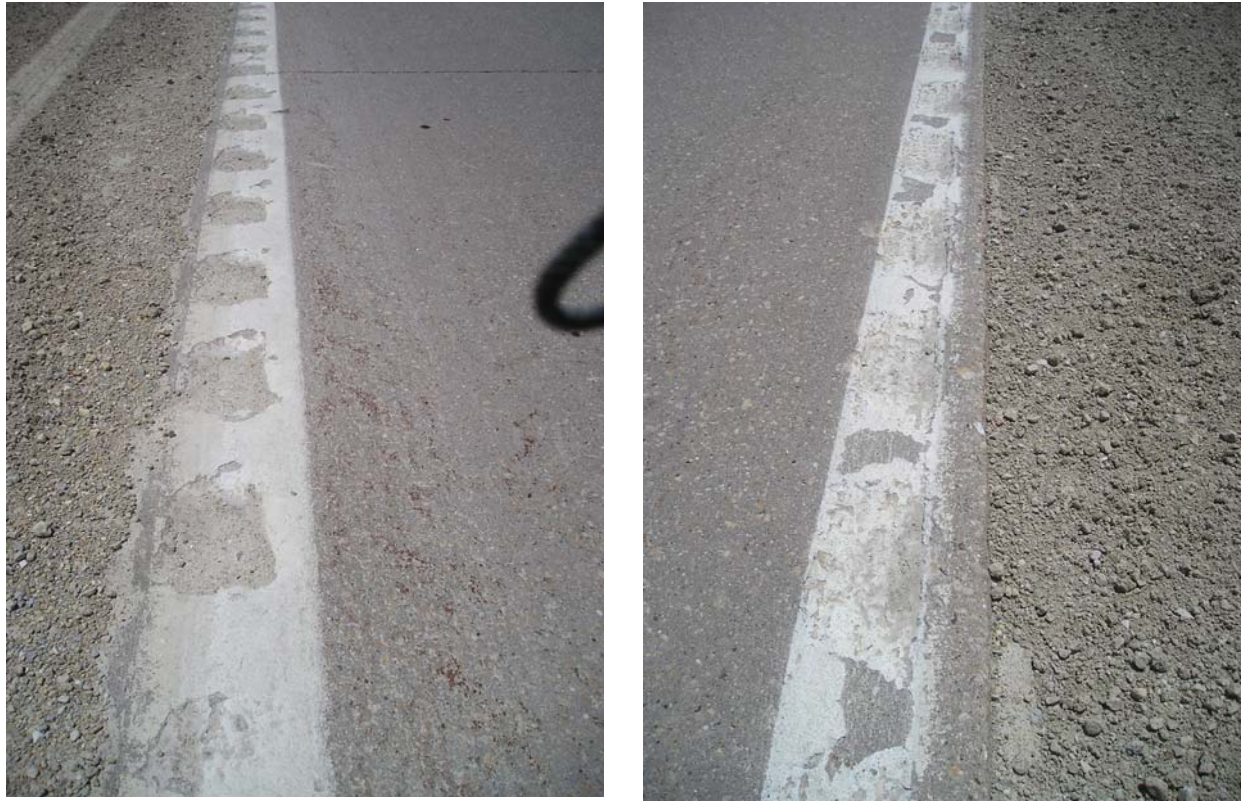
Figure 5-13. W-13 pavement markings in spring and after wear over winter, showing more wear in the groove than in the flat section
