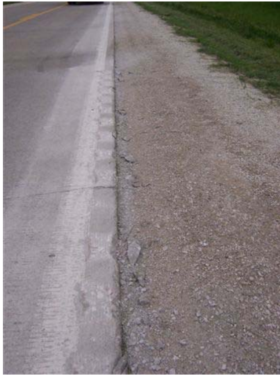
Figure 3-12. Edge spalling along edge of PPC pavement
