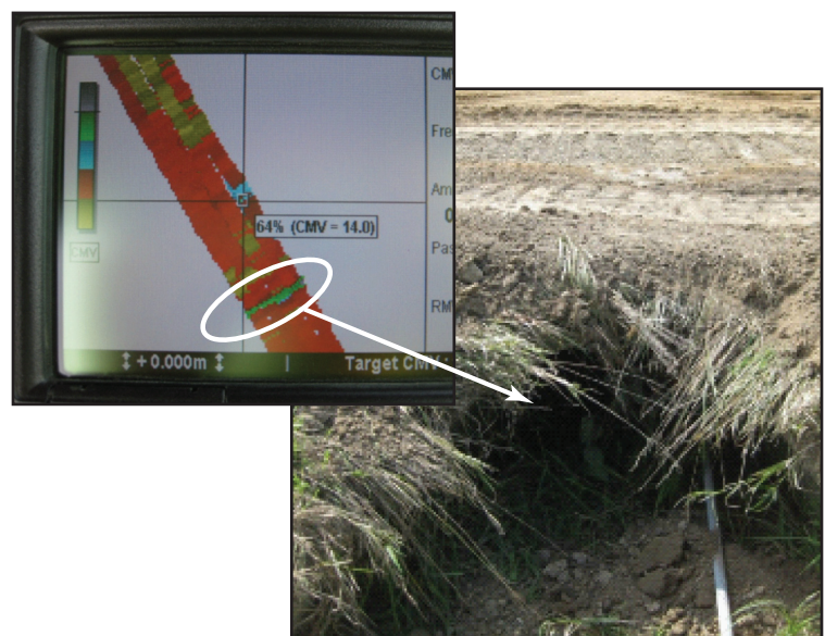
Figure 7. CMV map on an on-board display highlighting a box culvert location with a high CMV (from White et al. 2010)
