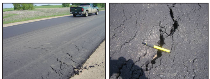
Figure 5. Premature failure observed in the HMA non-wearing course layer between Sta. 140+12 and Sta. 142+61 (from White and Vennapusa 2008)
