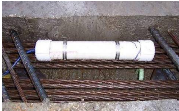
Figure 88. Vibrating wire gage with PVC pipe cover
