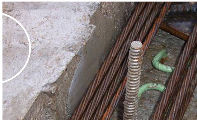
Figure 86. Concrete obstruction in Channel 1
