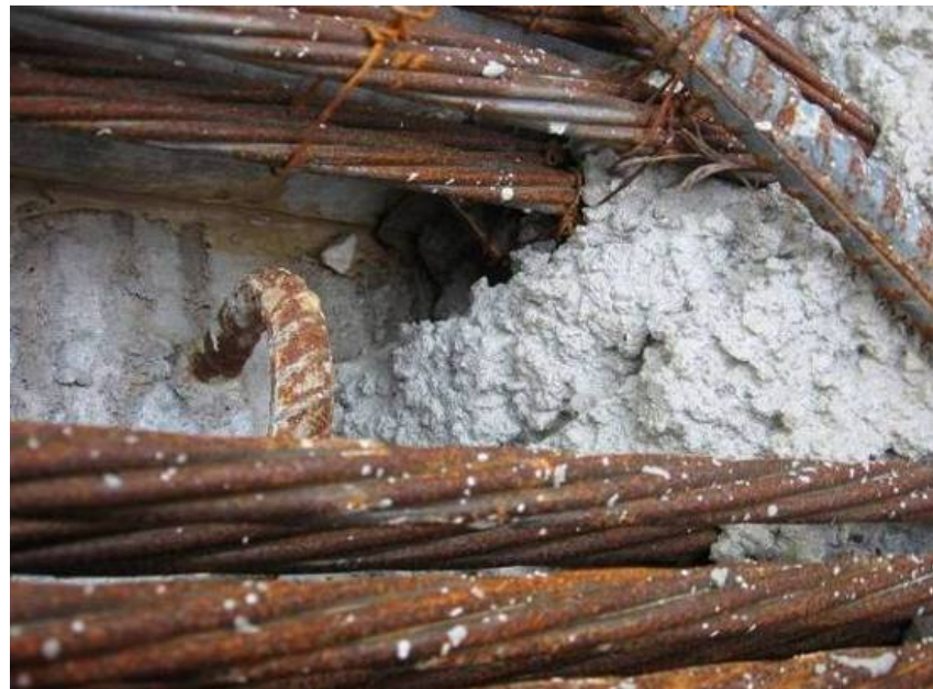
b) Concrete flowing between post-tensioning strands
