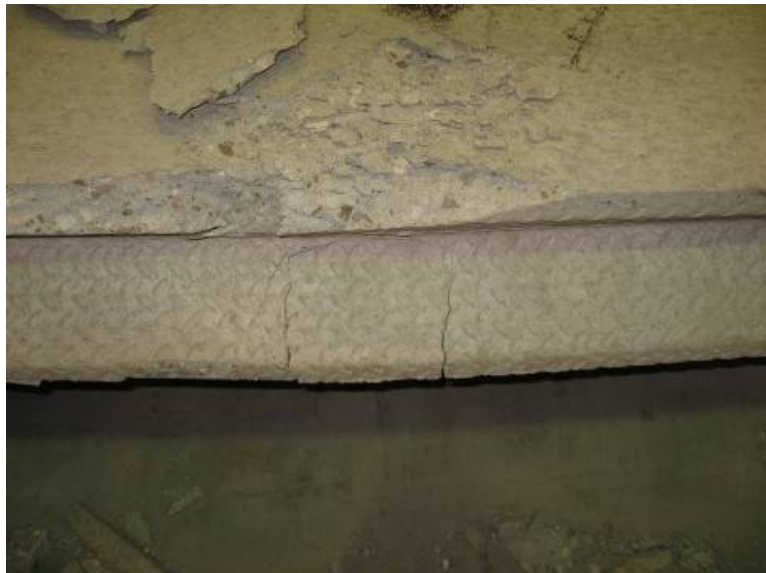
b) Flexure cracks
