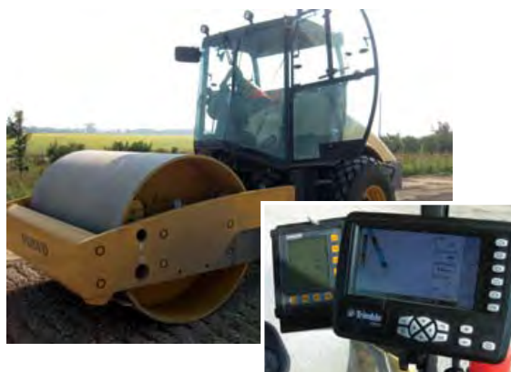
Figure 1. Volvo SD116DX smooth drum vibratory roller (top), and the on-board Trimble CB430 display (bottom)
