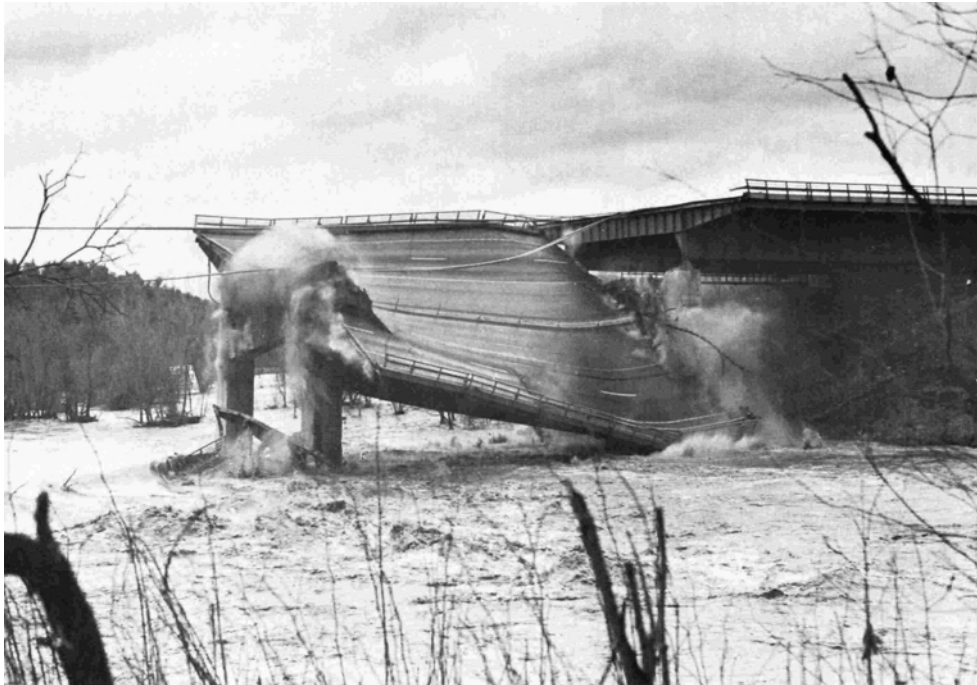
Figure 2.1. Photograph of the Skoharie Creek Bridge collapse, 1987
