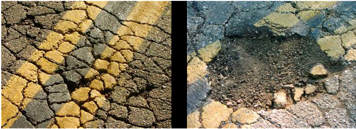
Figure 2. Alligator cracks and pothole formation
