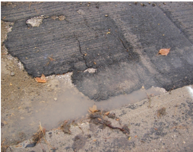
Cracks on temporary patch covering city practice trench indicating settlement (collapse) due to rain
