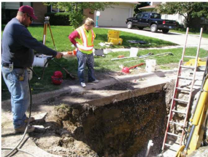
Watering backfill material to increase the moisture content beyond the bulking moisture content
