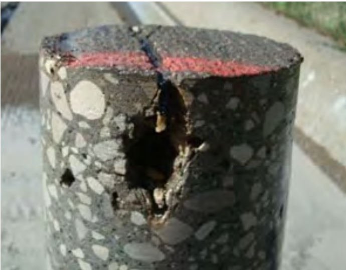
Figure 21. Joint deterioration evident below the joint sealant
