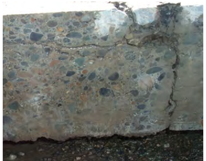
Figure 18. Example of delamination spalling (Source: Washington State)
