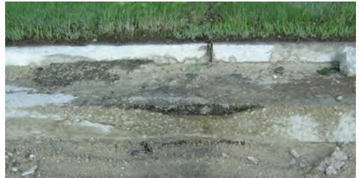
Figure 5. Typical saturated foundations under a shadowed section (Source: Snyder and Associates)
