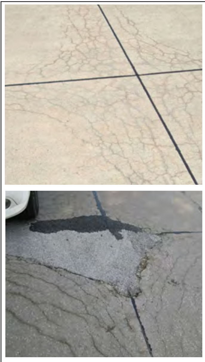
Figure 16. D cracking of low severity (top) and high severity (bottom) (Source: The Transtec Group)
