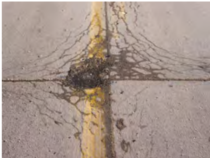
Figure 22. Deterioration due to D cracking
