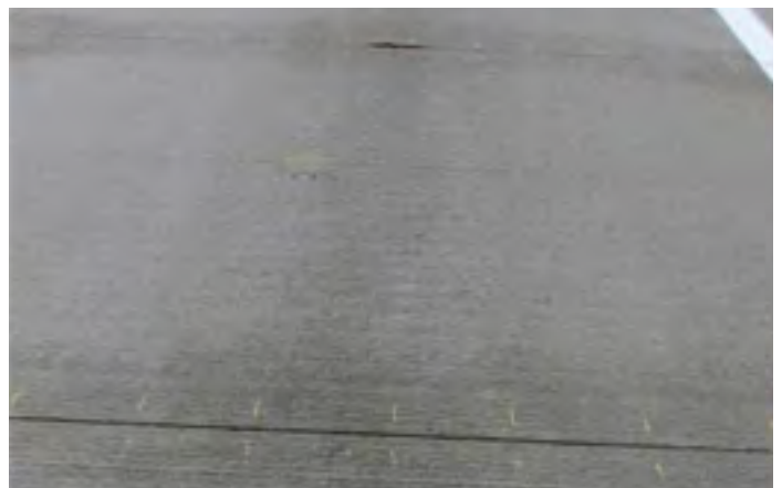
Figure 19. Shadowing at the joints, which is commonly followed by loss of material
