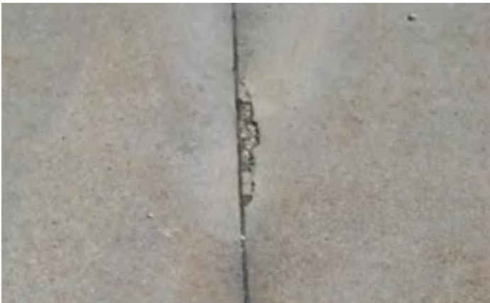
Figure 8. Water flow through joints from a high water table (bottom-up moisture); note staining on surface
