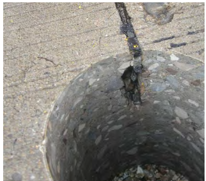
Figure 31. Evidence of saturation within joint beneath seal (Source: Purdue)
