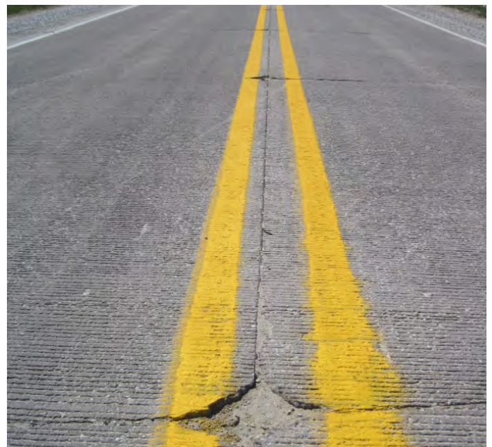
Figure 25. Damage starting at joint intersections
