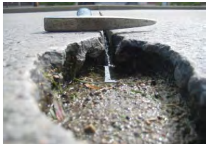
Figure 27. Example of a poorly draining pavement
