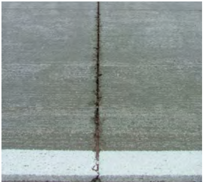
Figure 24. Joint deterioration due to raveling from improper saw-cut procedures
