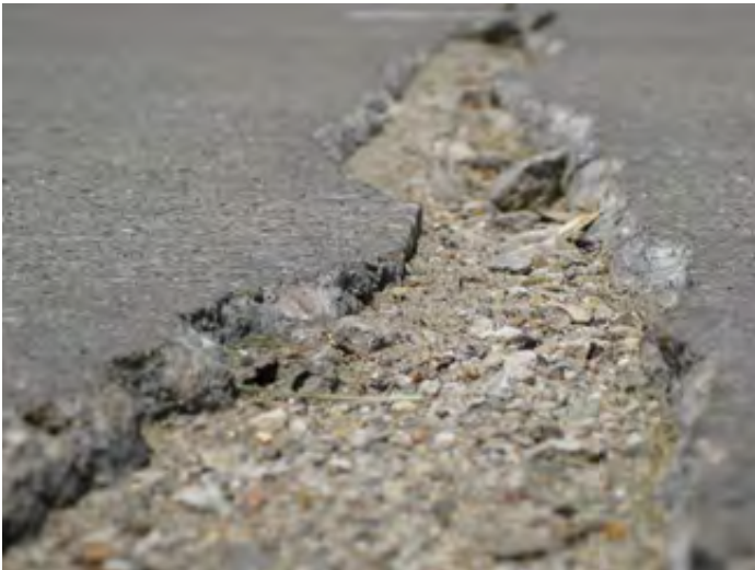
Figure 20. Top-down joint distress, with vertical edges and shallow depth
