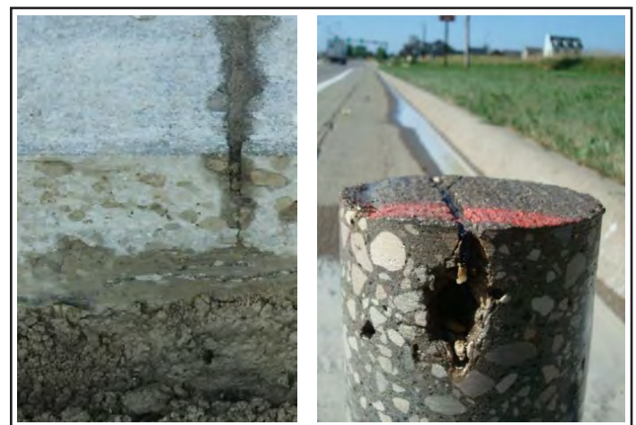
Figure 3. Saturated soils due to inadequate drainage and roadside irrigation (left) leading to joints showing frost damage (right) (Source: Snyder and Associates)
