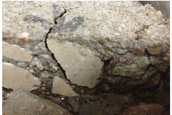
Figure 12. Photograph of a crack around an aggregate particle
