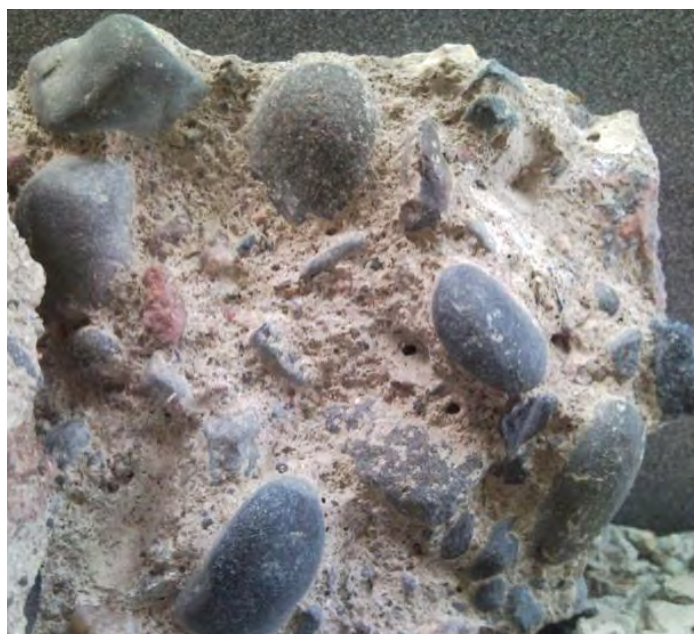
Figure 10. Coarse aggregate exposed by damage to the paste
