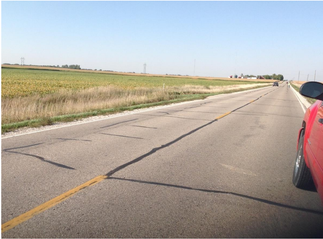
Figure 57. Performance condition on G61 (East) project
