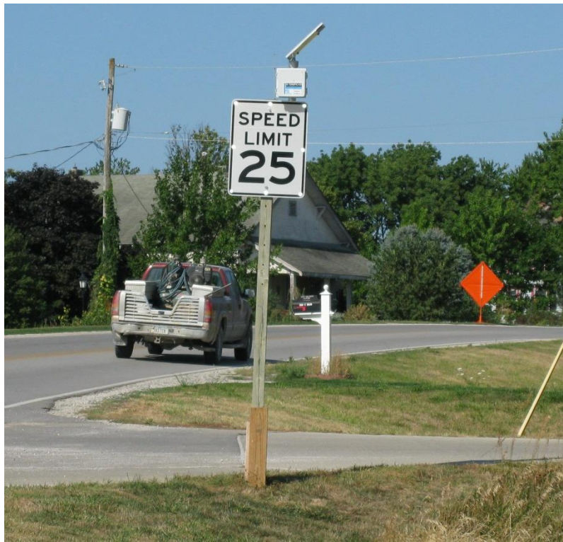
Figure 52: Speed limit sign with radar-actuated LEDs around the border
