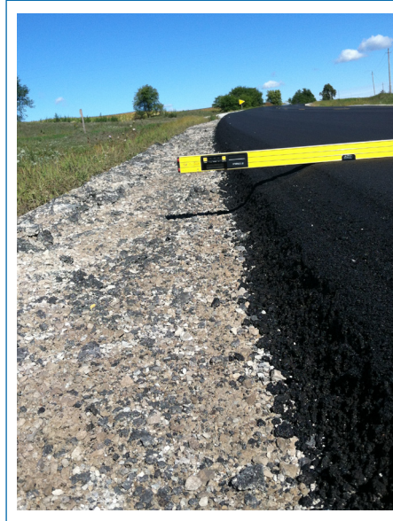
Figure 4. Severe pavement edge drop-off near outside of curve
