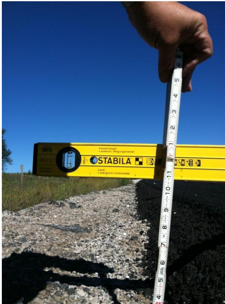
Figure 15. Severe pavement edge drop-off
