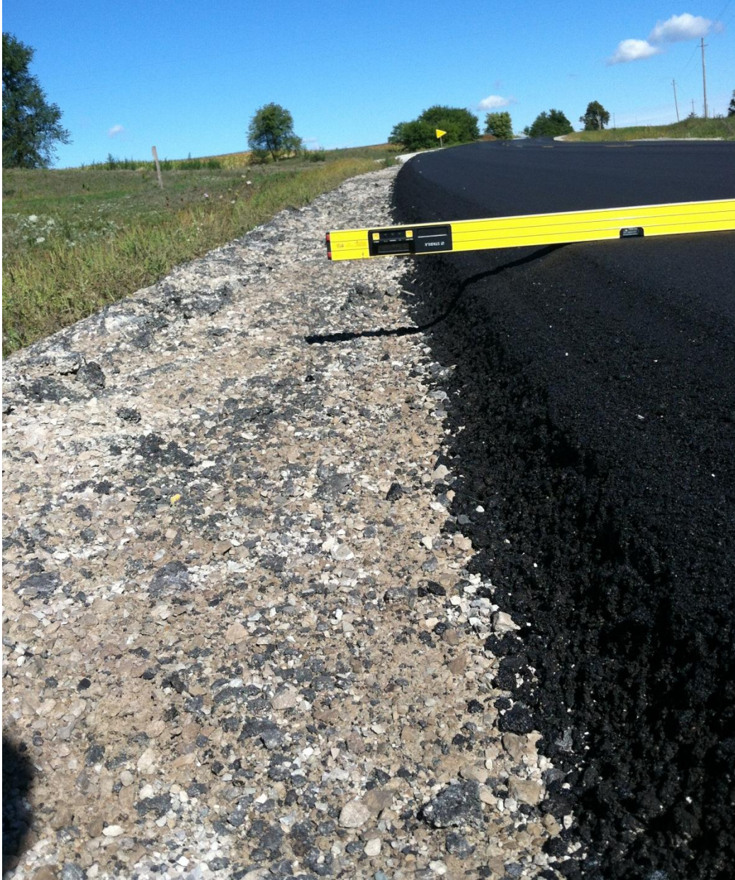
Figure 14. Severe pavement edge drop-off near outside of curve
