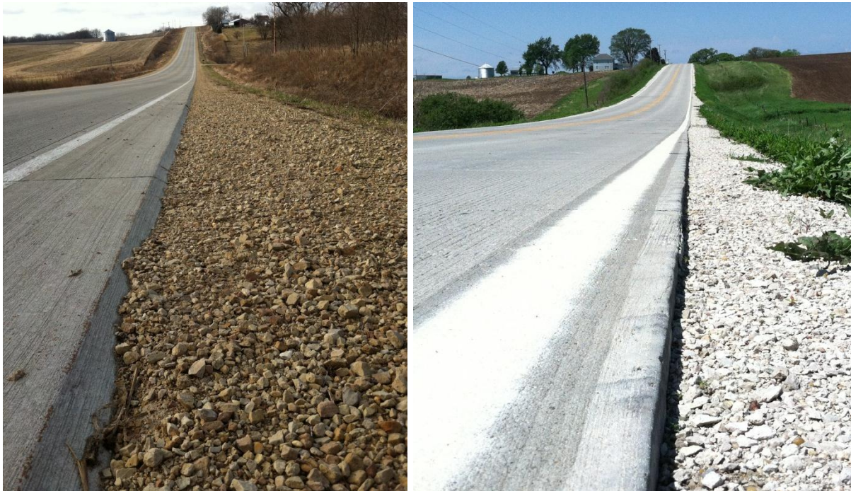
Figure 9. Typical shoulder degradation for PCC pavements with the Safety Edge (left) and without it (right)
