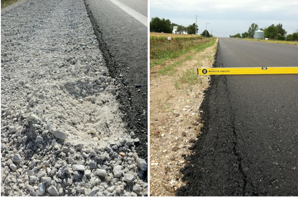
Figure 11. Edge cracking from apparent lack of shoulder support
