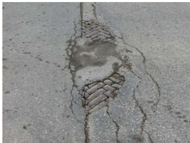
Deteriorated asphalt surface with exposed brick
