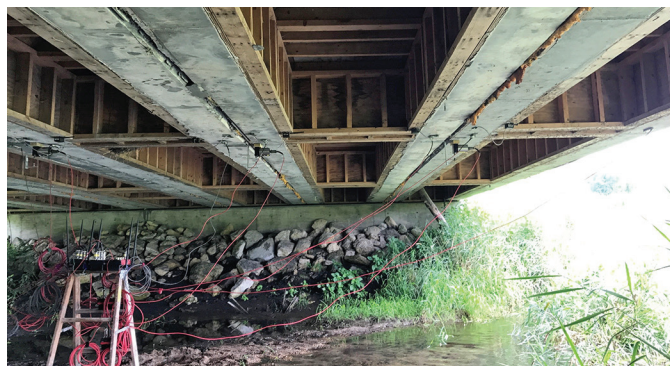
Instrumentation of the precast girders for live load testing two years post-construction
