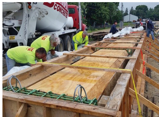
Formwork for pouring and casting the K-UHPC cross-section pi-girders in the Buchanan County Secondary Roads yard
