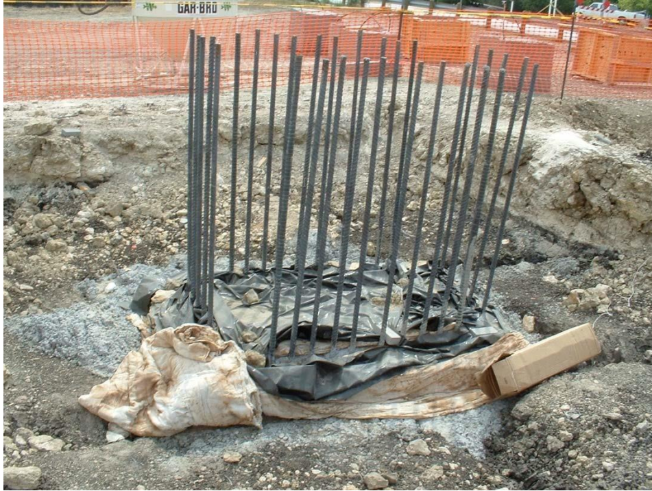
Figure 8 - Example of a footing that would use the “soil on the sides” option
