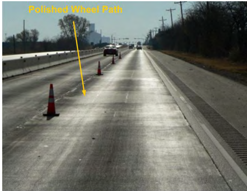
PCC pavement made with 100% limestone sand showing polishing in wheel paths
